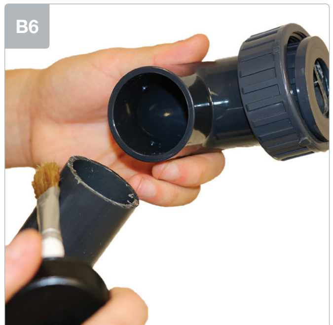
Using high pressure PVC glue, apply to both the discharge arm and the inside of the 90° bend. Push and twist the components together to expel any air - allow to cure.
